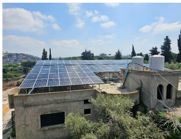
Qaaqaiet El Sanawbar Solar System- roof 2
