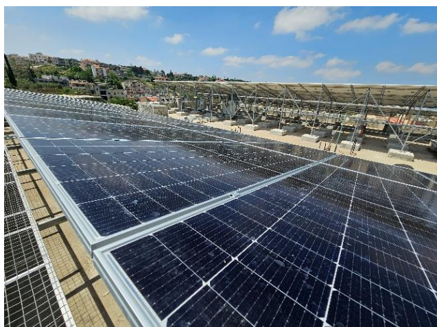
Qaaqiet El Sanawbar Solar System- roof 1
